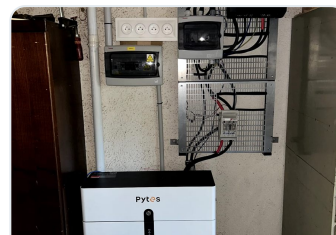
Exploitation &amp; stockage
